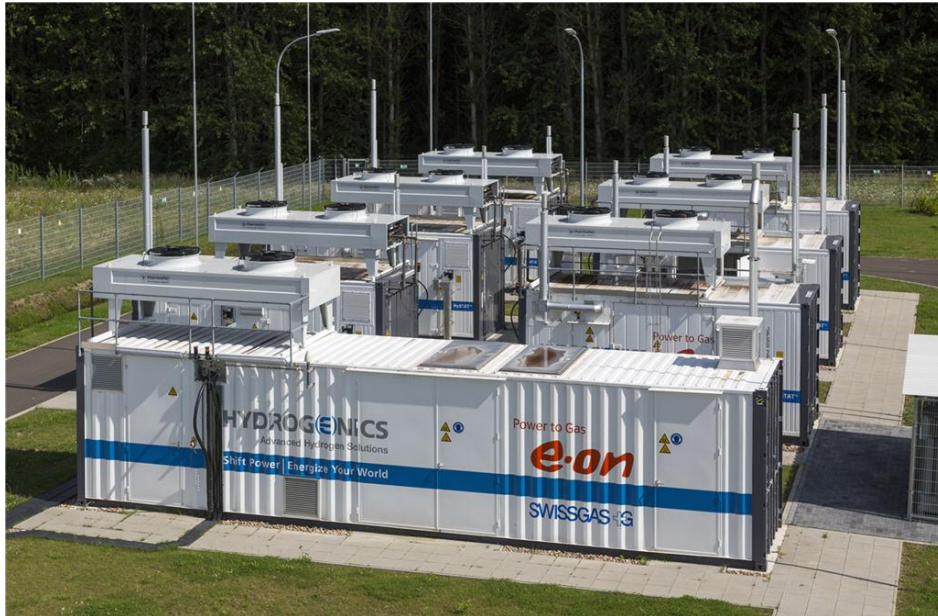
Figure 17 – Le système Hydrogenics/StratosFuel de 2,5 MWe (2016)
