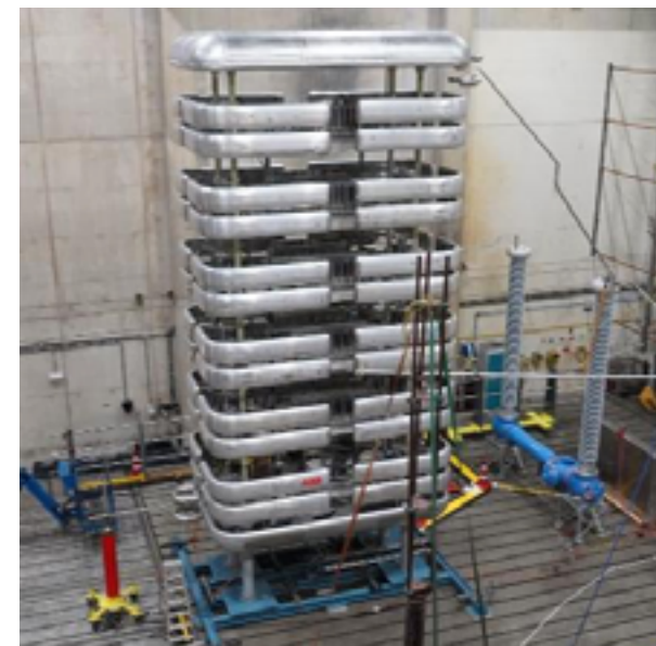
FIGURE 7. Demonstration of HVDC circuit breaker performance in the KEMA Lab’s high-power laboratory during PROMOTioN project
