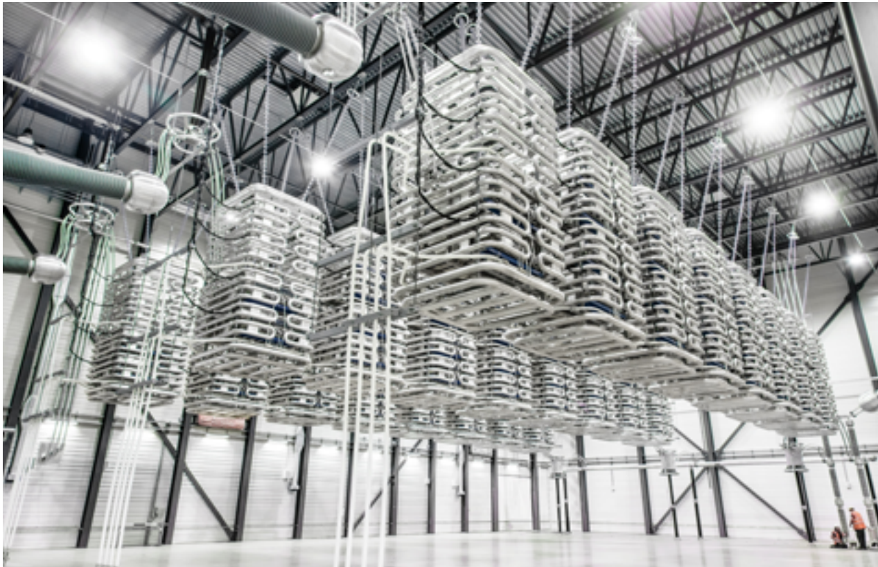
FIGURE 6. HVDC Light Valve Hall
