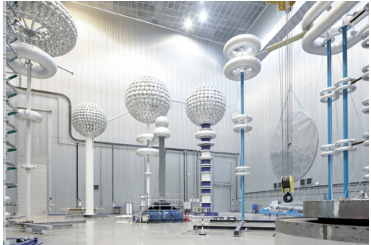
FIGURE 3. Hitachi Energy's ultra high-voltage test hall in Ludvika, Sweden, where the highest voltage products are tested for both AC and HVDC projects.
