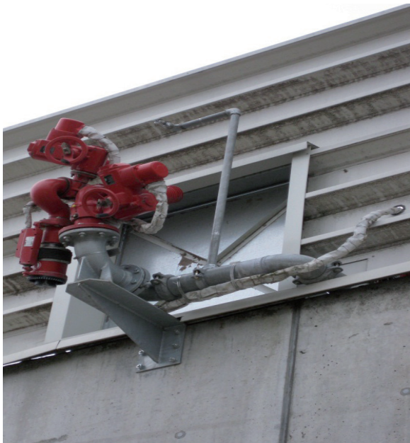
Figure 3.13. Example of a remote controlled water cannon installed on the capstone of a fuel storage facility for a first fire extinguishing [86].
