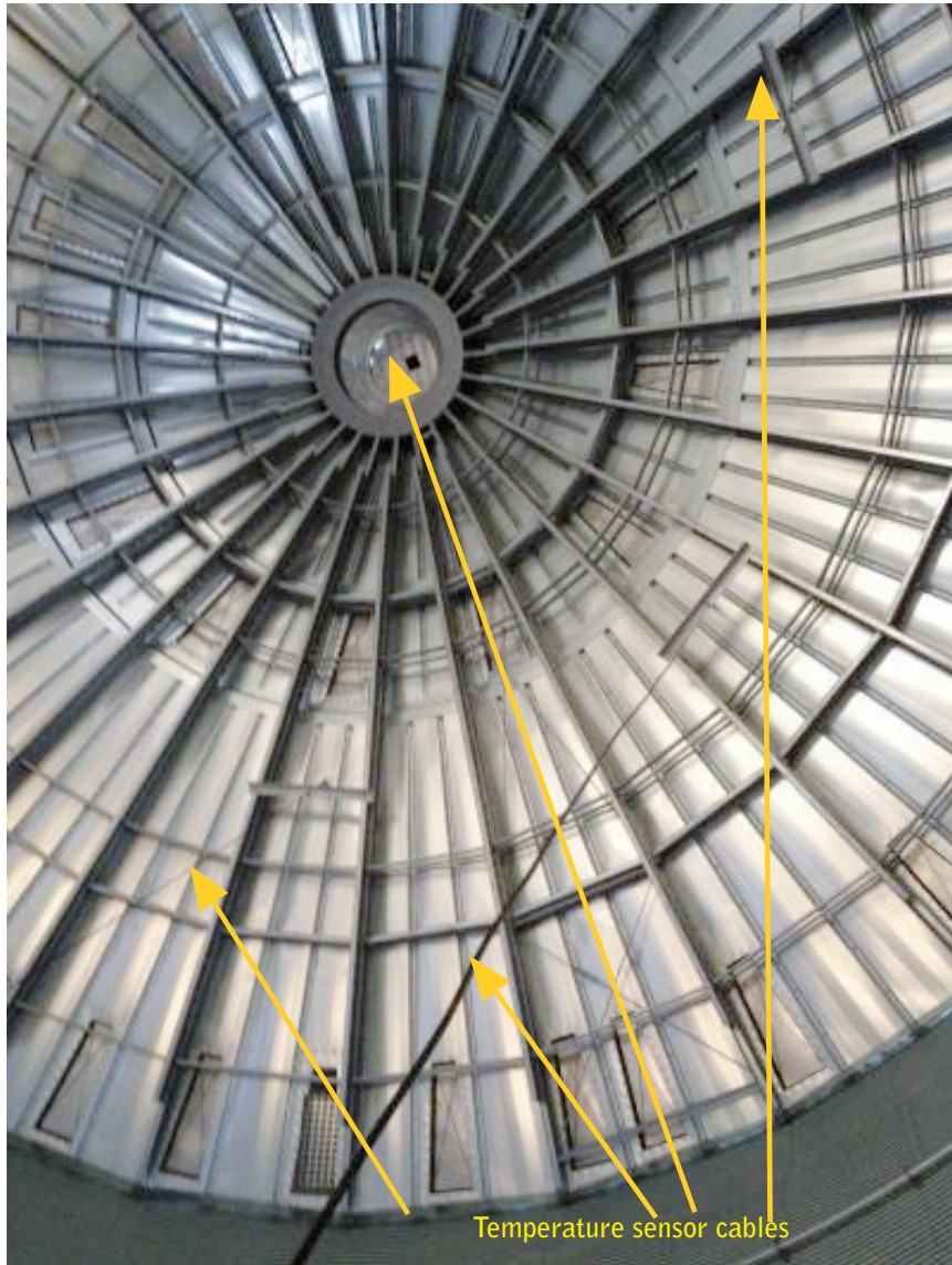
Figure 3.16. Monitoring of the temperature trends inside bulk storage is important to indicate if there is an unusual self-heating on-going. The black lines from the roof in the picture show temperature sensor cables normally used for such monitoring. This silo (20 m in diameter) is equipped with one line in the silo centre and six lines distributed at half the radius. All together the seven lines include 37 temperature sensors which are connected to a control system. (Photo Anders Lönnermark, SP)
