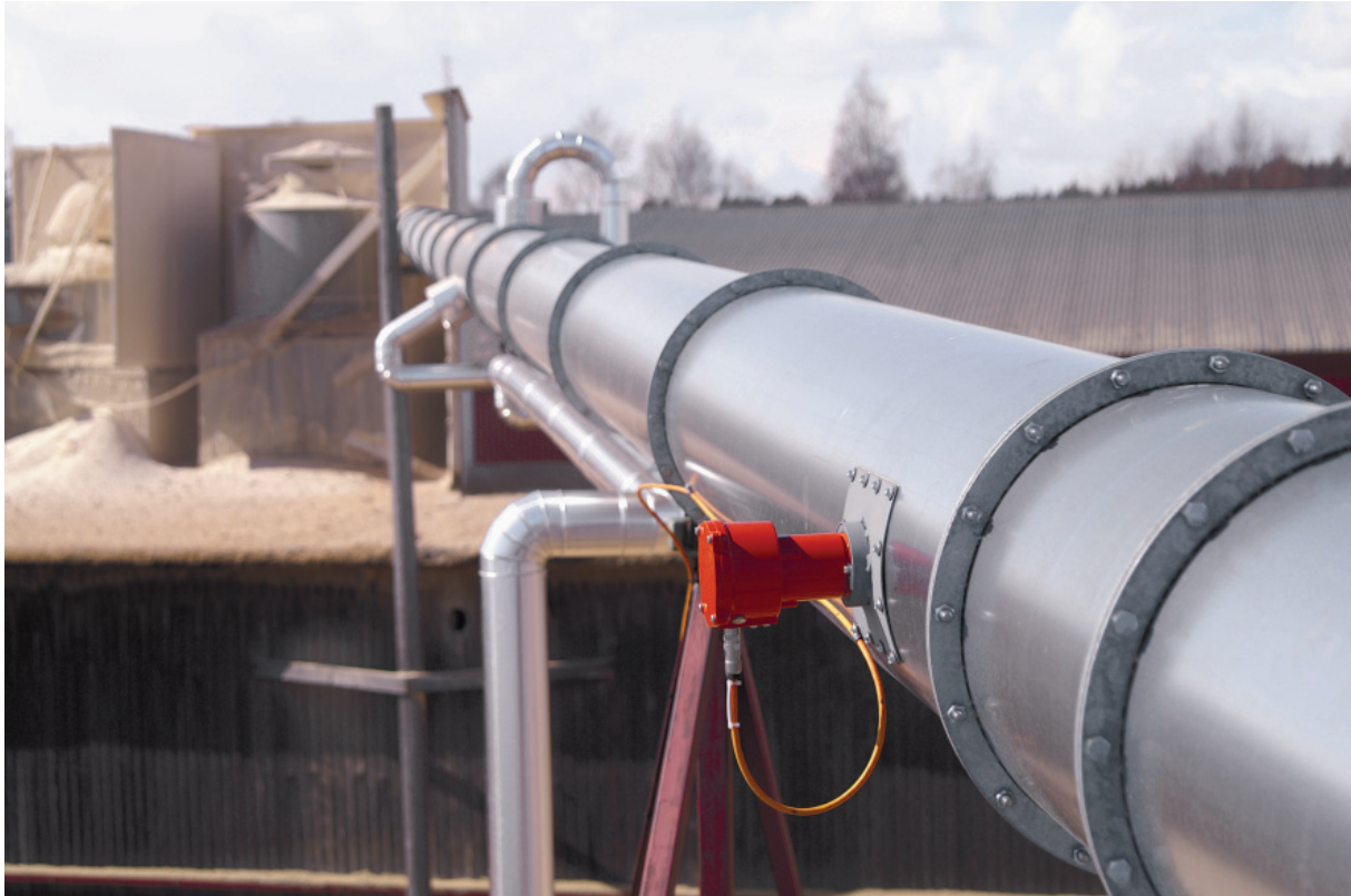
Figure 3.8. A detector indicating sparks and hot particles in a ventilation duct. These detectors are often connected to a fast activating water spray system downstream the detector (not in this picture) (courtesy of Firefly).
